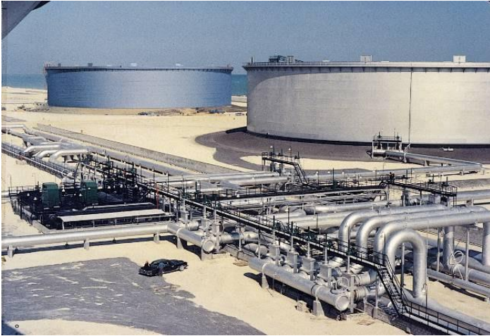
Fig. 4: Oil and Gas Pipeline Network with Welded Joints
