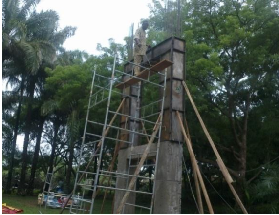
Plate 3a: The two-leg reinforced concrete tower of the Suspended Walkway, designed and construction supervised by me in 2012
