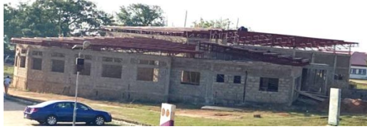
Picture 10: Batuli Ajiferule Shagaya Burn Intensive Care Unit (BICU), UITH Ilorin, under construction
